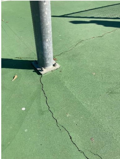
Light Pole Base (COURT 8)
